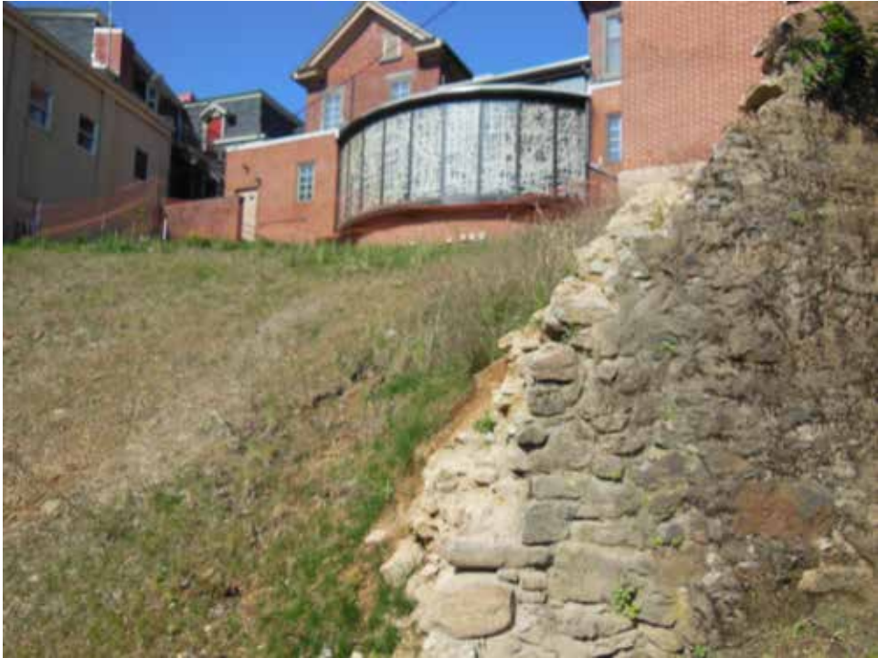
Image 21: Image of collapsed stone retaining wall on site looking from east towards west; Image taken by Spillman Farmer on April 11, 2023.
