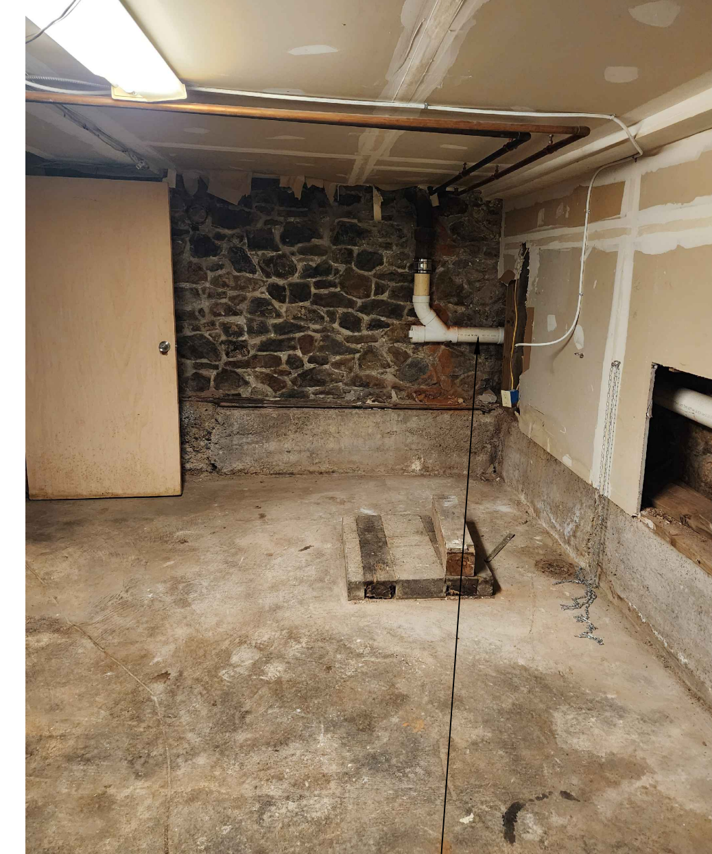
EXISTING MAIN PIPES TO REMAIN. ALL BRANCHES SHALL BE REMOVED AND CAPPED.
