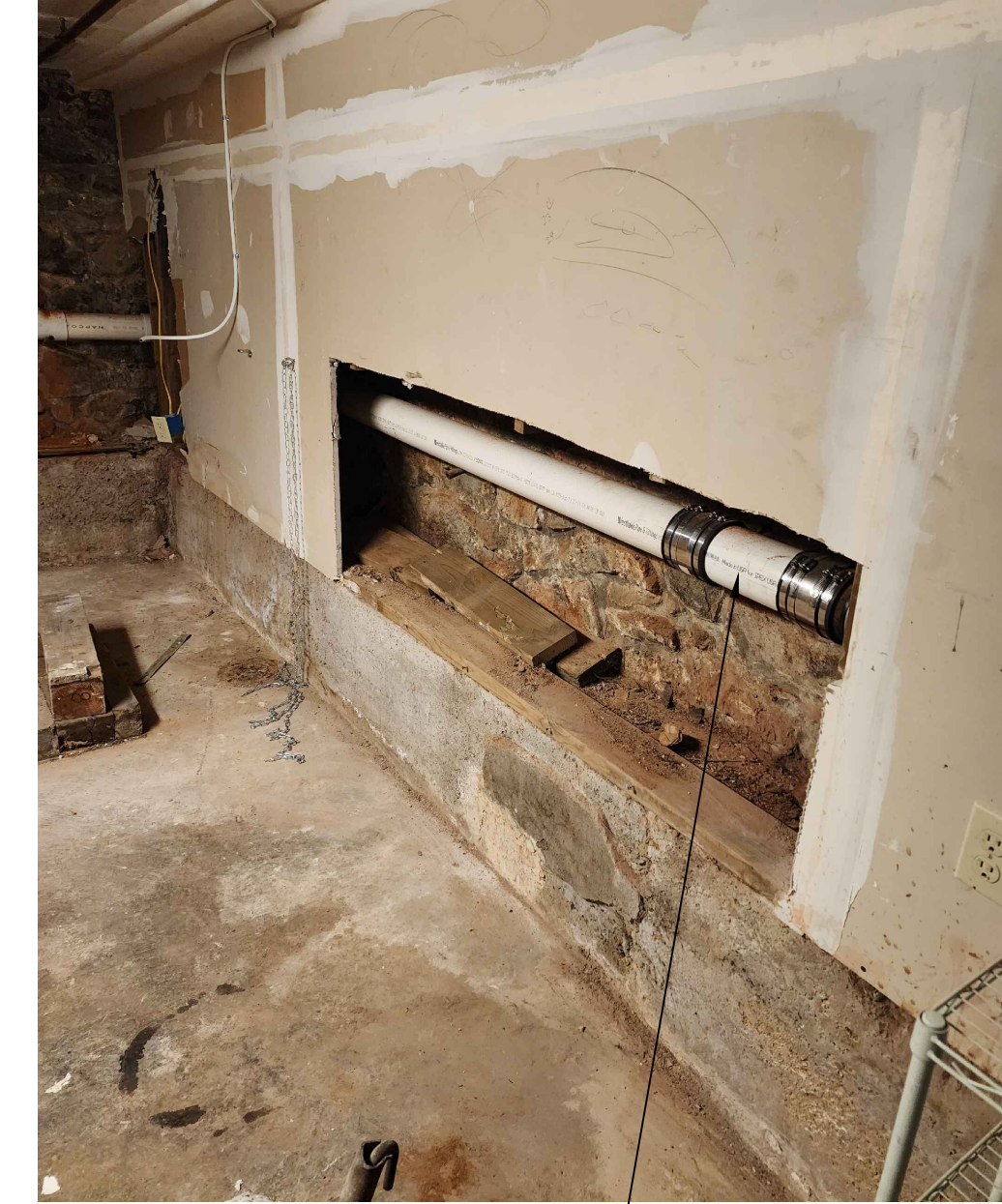
EXISTING MAIN PIPES TO REMAIN. ALL BRANCHES SHALL BE REMOVED AND CAPPED.
