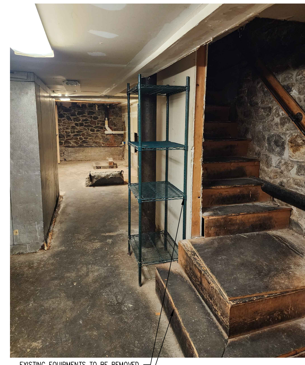
EXISTING EQUIPMENTS TO BE REMOVED STAIRS TO BE REPAIRED AS REQUIRED
