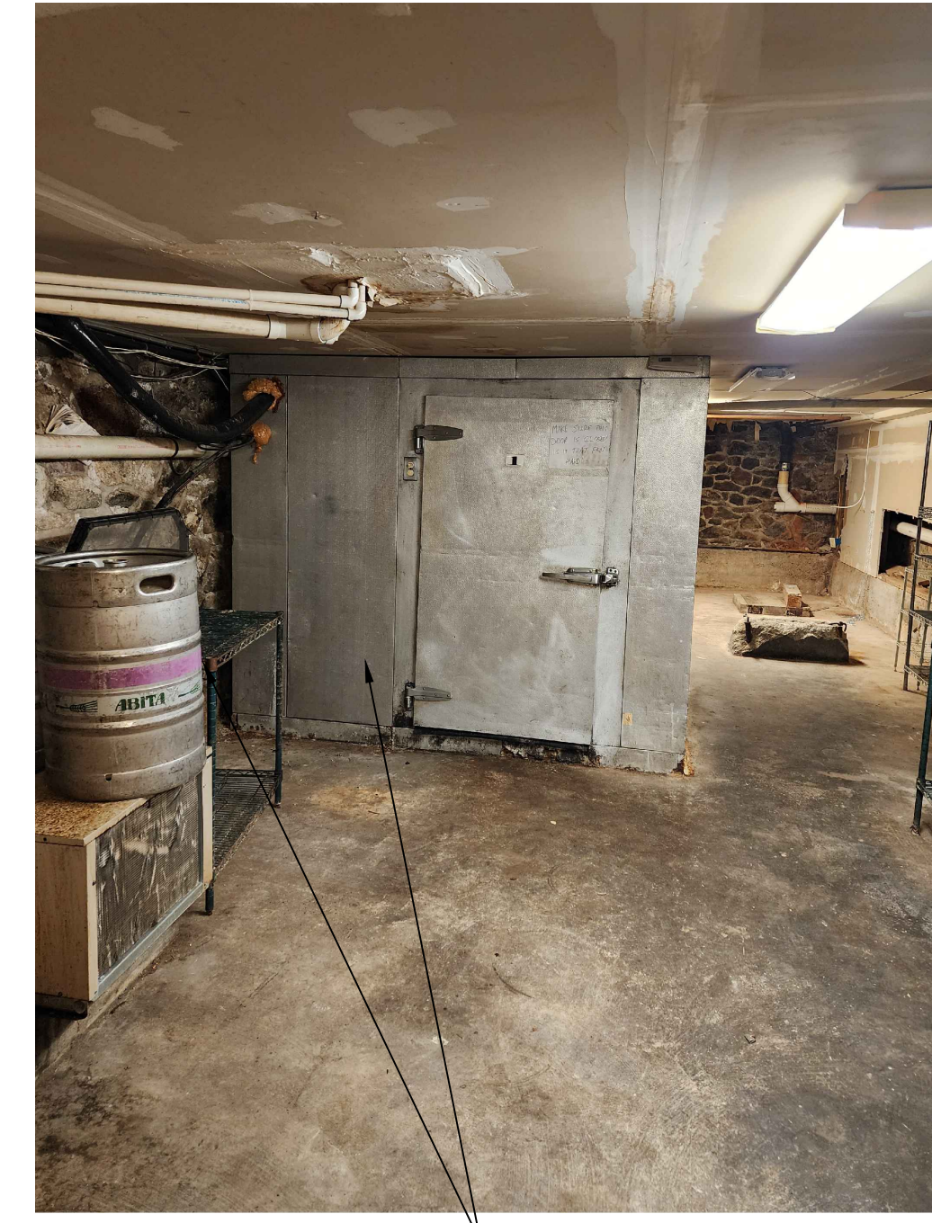
EXISTING EQUIPMENTS TO BE REMOVED
